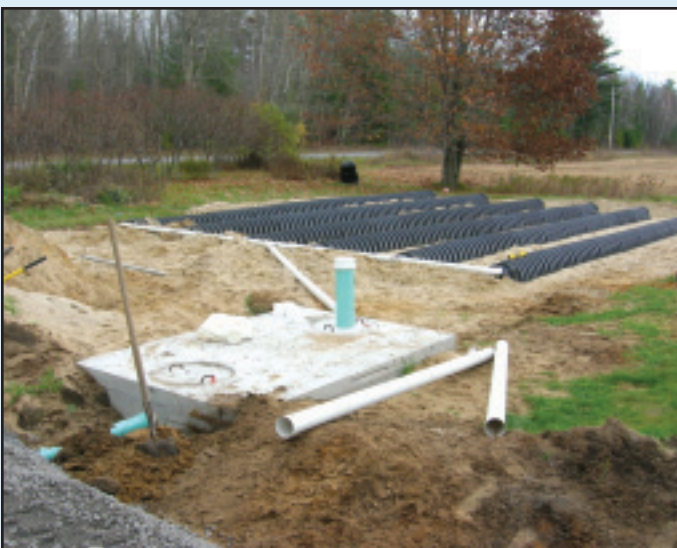
Leaching bed with gravelless trench technology.
