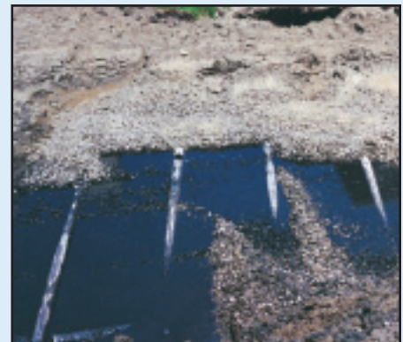
A failed system exposed.
