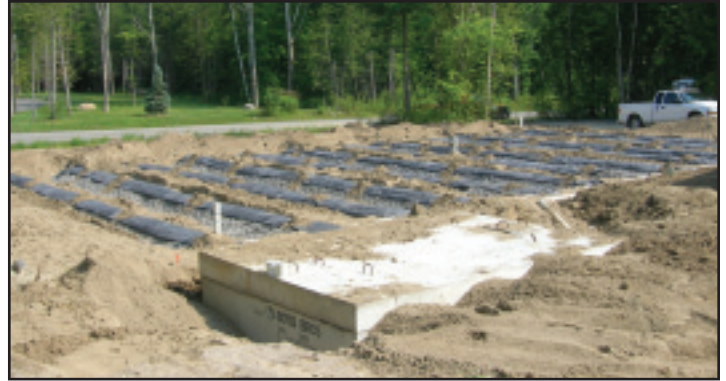
Septic tank and leaching bed.
