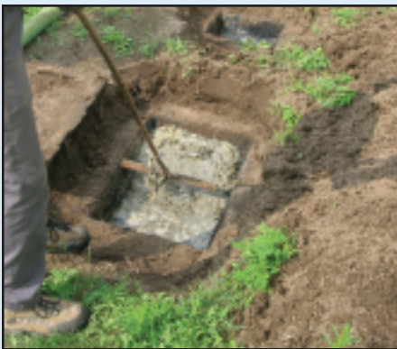
Scum level is too high. Time to pump your tank and inspect your leaching bed.
